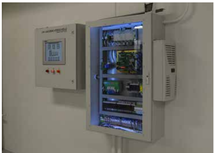
The Capstone tri-generation system provides the facility with baseload electricity, hot water, chilled water, and backup power in the event that the local utility goes down
