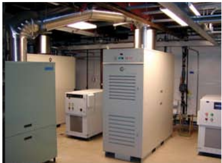
Capstone microturbines generate electricity, cooling, and heating at Vineyard 29 in Napa Valley, California.
