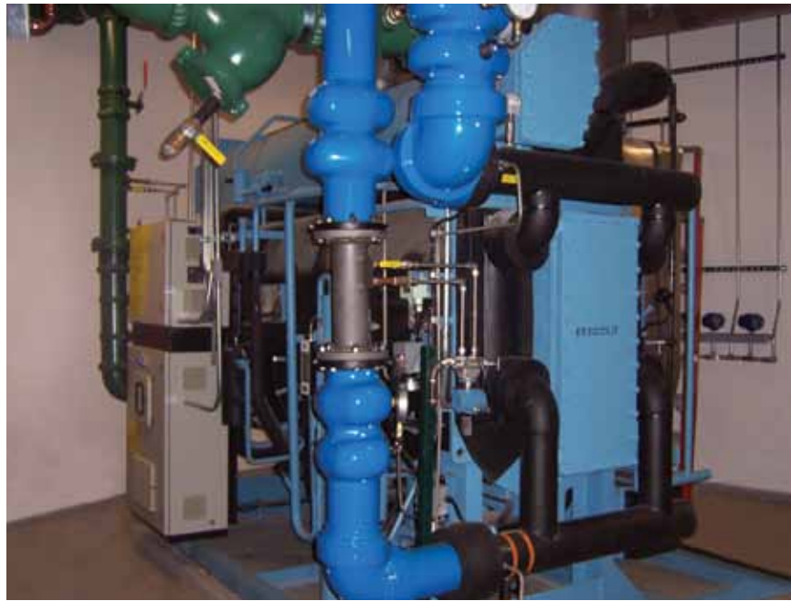
Thermax® absorption chillers.
