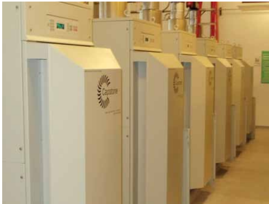
Twelve Capstone C65 Hybrid UPS microturbines are installed in Syracuse University's Green Data Center. The center is designed to use 50 percent less energy than traditional data centers.
