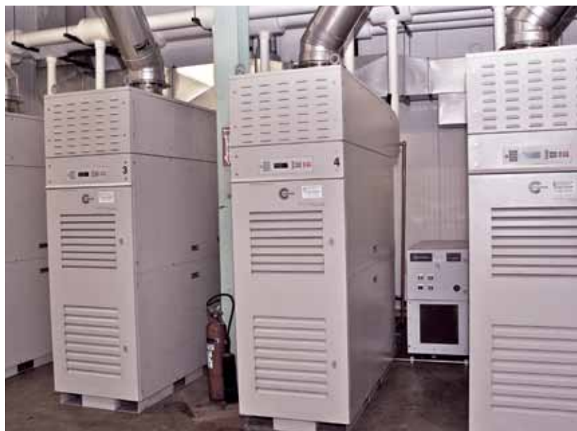
Capstone microturbines provide cooling, heating, and power at Astor Chocolate in New Jersey.
